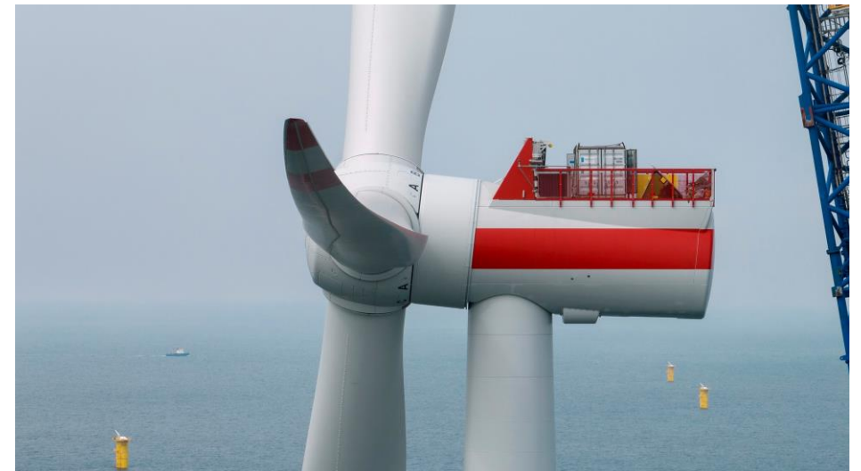
RWE installed the world's first recyclable wind turbine blade manufactured by Siemens Gamesa.
